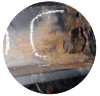
Corrosion of the existing floodgates
